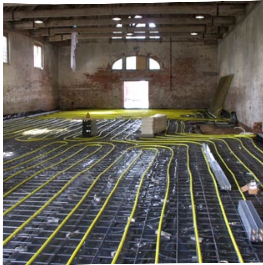
Above Under floor heating to Riding School
